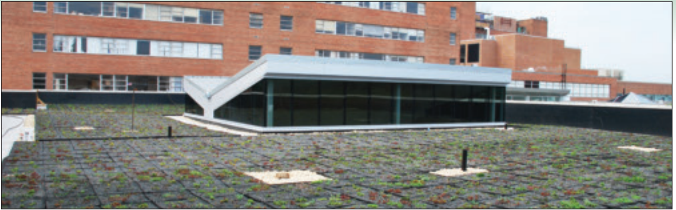
A section of the massive green roof installed at Sibley Memorial Hospital in Washington, DC.
