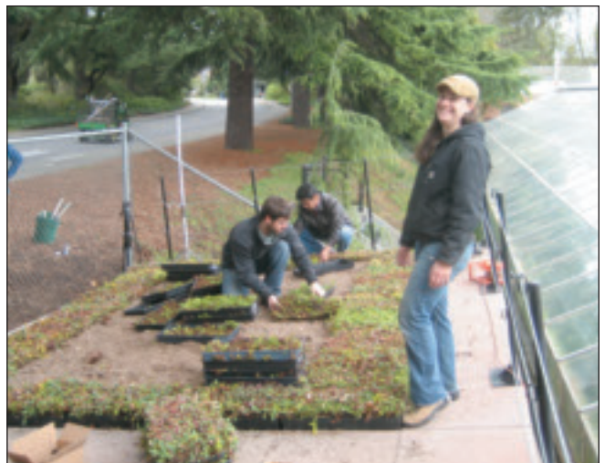
University of Washington students plant specially selected plants on the experimental green roof.
