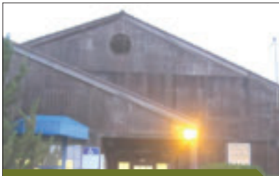
Before the renovation, the Rio Vista Senior Center had damaged wood siding for an exterior.
