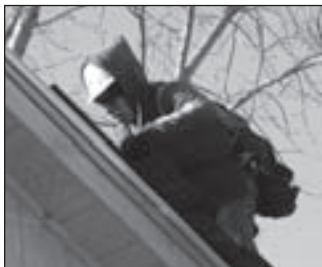
Brother Huber nails down the shingles donated by Prate Installations, Inc. of Wauconda, Illinois.
