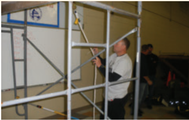
Trainers learned how to attach PFAS to anchors without exposure to fall hazards. Chris Milliron, Roofers Local 44, Cleveland, OH, practices his technique.
