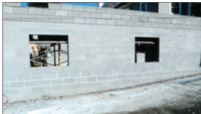
The beginning stage of construction on the Local 188 training facility shows just the concrete block exterior.
