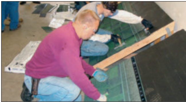
Third-year apprentice Vladamir Petrushyn (front) and second-year apprentice Will O'Brien hand-nail to perfection in the steep-roof contest.
