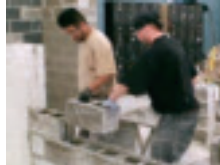
Workers use the two-mason lift technique to reduce stress of lifting and twisting.
