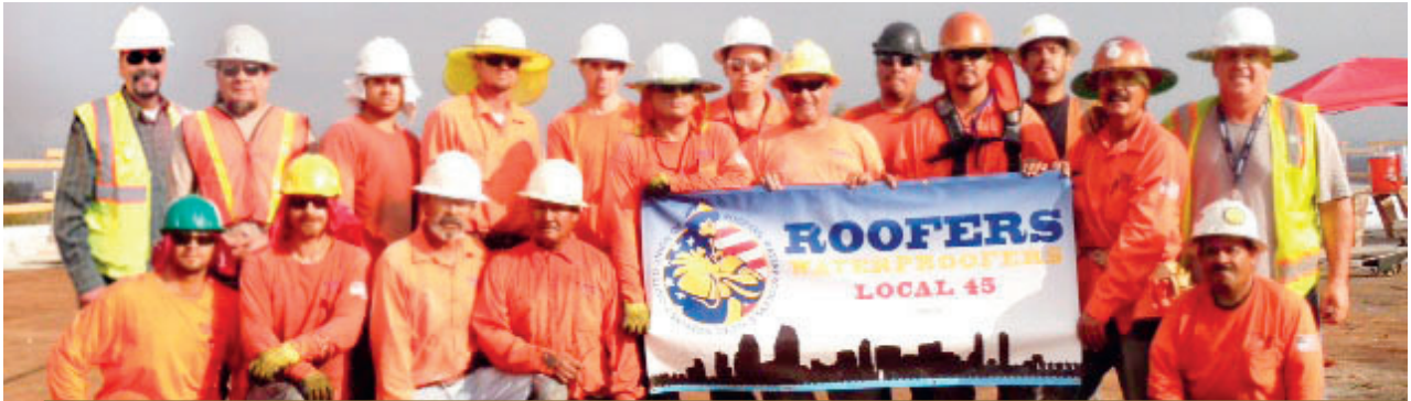
Re-roofing the Kaiser Permanente building in Kearny Mesa are (standing, from left) Local 45 Rep. Paul Colmenero, Market Development Rep. Raul Galaz, Juan Campos, Daniel White, Jessie Chambers, Jesus Quevedo, Adam Chambers, Jesus Aguilar, Ruben Alcaraz, Miguel Gasca, Robert Hernandez, foreman Bobby Colmenero and Ron Chambers, owner/president of Roof Construction. Front row: Nicholas Jimenez, Brendan Vannie, Roy Sugioka, Marcelino Percastegui and Victoriano Palacio.
