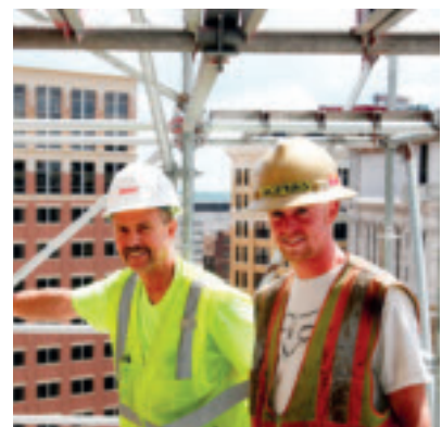
Mark Anderson (father) and Eric Anderson (son) of Dalco Roofing are the father-and-son team installing tile on the Landmark Center.
