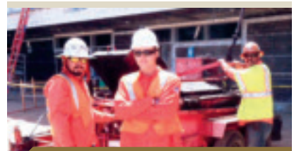
Roof Construction employees Miguel Cuevas, Adam Chambers and foreman Bobby Colmenero roof National City Middle School.
