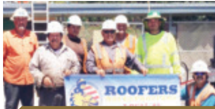
Jose Perez, Jesus Felix, Jaime Moreno, Simon Medina, Tab Rapp, foreman Eddie Stopani and Wayne Lawler, who work for A Good Roofer, roof Hearst Elementary School in the Del Cerro neighborhood.
