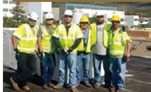
Local 123 members Rocky Lopez, Joseph Fernandez, Rocky Madrid, Floyd Cordova, Jose Maestas and Johnny Quintana perform roofing on Los Alamos National Lab.
