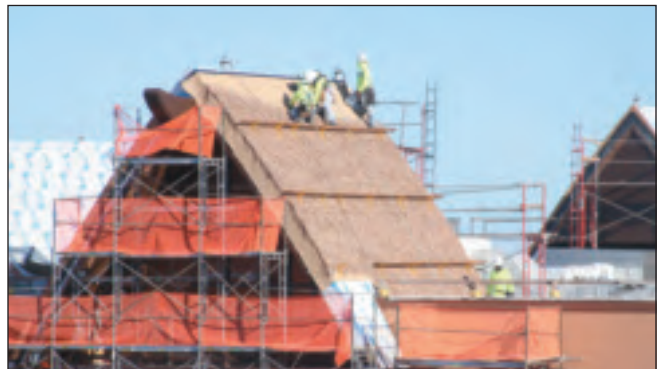
Local 221 employess of Beachside Roofing in the process of laying thatch product on the Disney Aulani Resort.
