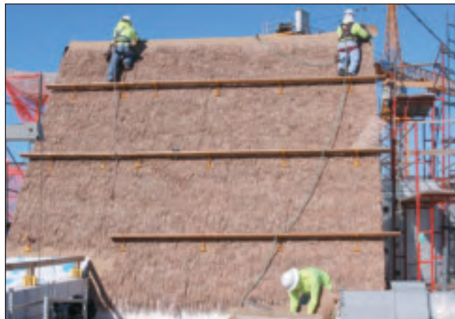
Local 221 roofers apply a faux-thatch finish to the structures at Aulani Resort.
