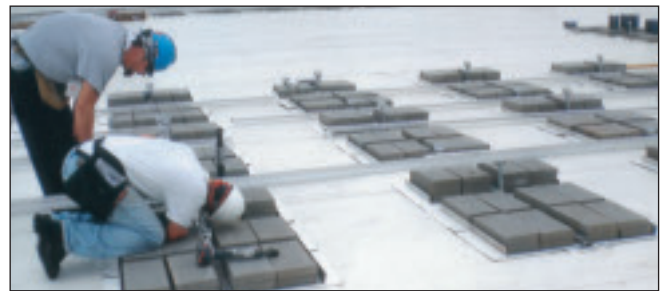
Local 10 and Local 30 roofers make minor adjustments to the pavers on the GlaxoSmithKline project.
