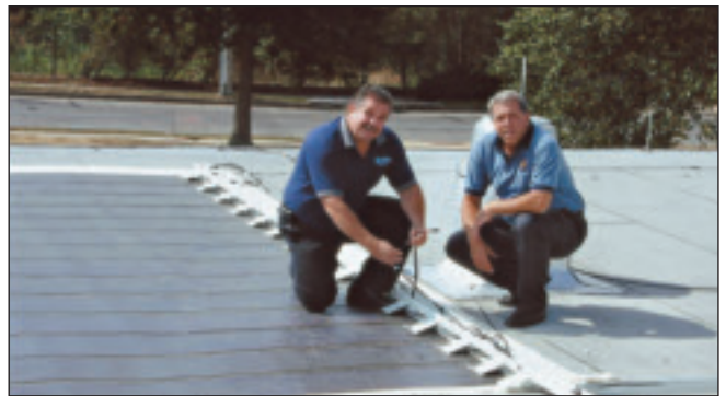
Local 154 Apprentice Instructor John Keating and Union Representative Sal Giovanniello inspect work.
