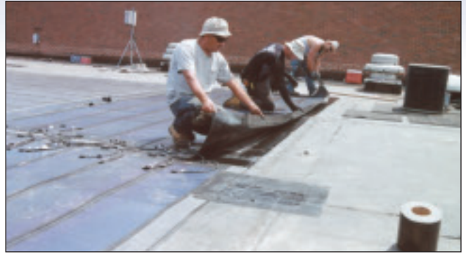
Paul Kelly of Local 154, Pete Milanese Jr. of Local 6 and Ron Hinklein of Local 154 apply solar membrane to a job at Bellport High School in the town of Bellport on Long Island, NY.
