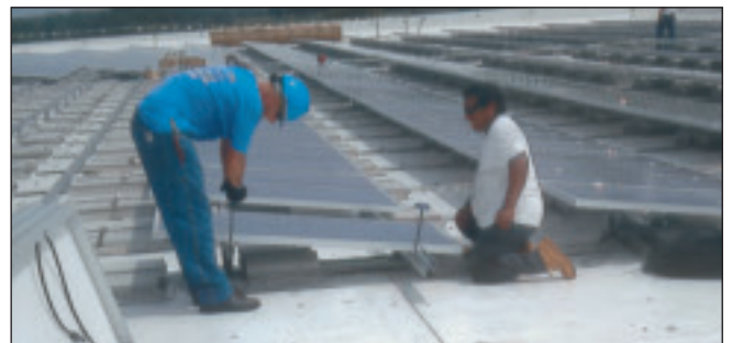
Employees of Patti Roofing check panels to make sure they are correctly integrated with the roof system.
