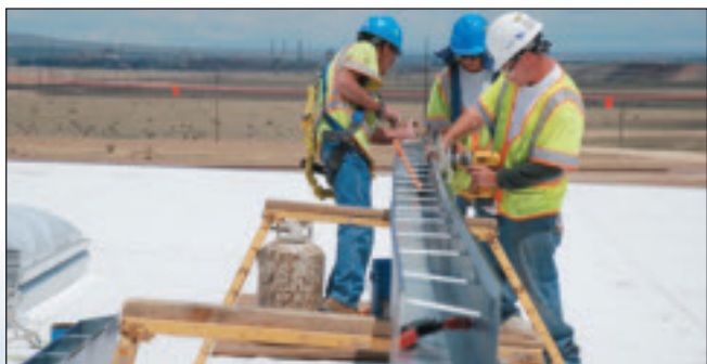
Local 58 roofers John Snyder, Rino Roussel and Miguel Estrada put the finishing touches on the Vestas roof.
