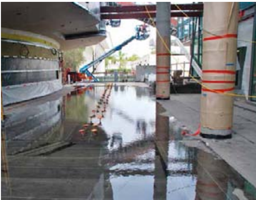
Water testing is conducted throughout areas of the Life Science building that have been waterproofed.
