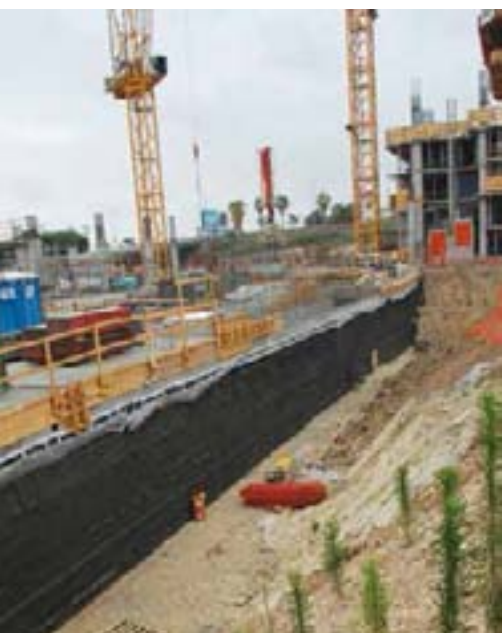
Troyer Contracting performs below-grade waterproofing on Metropolis, a luxury residential highrise in the South Park neighborhood.
