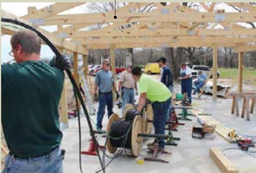
Building trades union volunteers build a new storage facility at H. Roe Bartle Scout Reservation in Osceola, MO.
