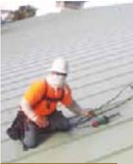
Protected from falls and from the sun, Honolulu Roofing employee Lucas Rosa works on the Aloha Tower roof on Honolulu Harbor.
