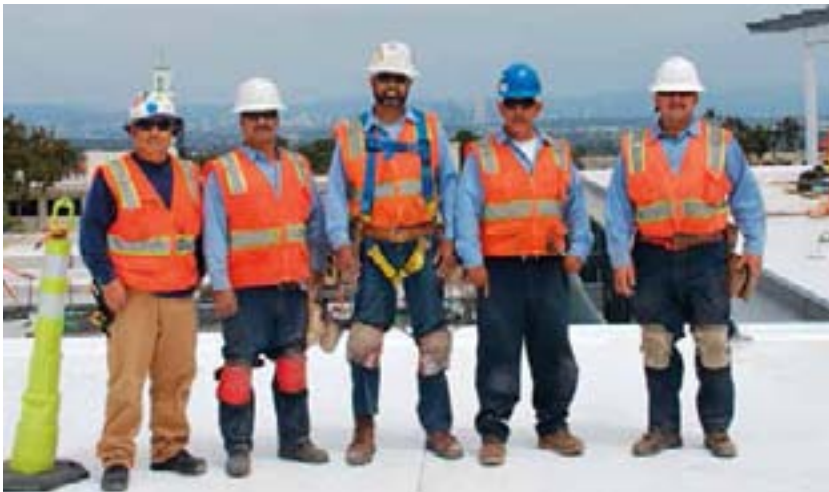
Local 36 Roofers Michael Mora (foreman), Luis Lopez, Joel Prieto, Jose Marquez and Victor Santana (single-ply foreman) roof the top of the Life Science building.
