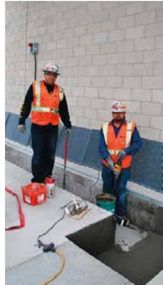
Arturo Lagunas (left) and Jose M. Rocha apply Xypex waterproof coating to a cement trough at the Bus Maintenance & Operations Facility.
