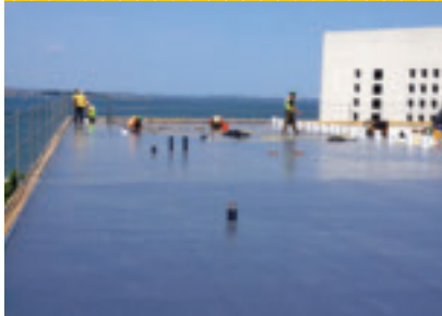
Roofers finish the roof on the Edward M. Kennedy Institute on UMass Boston campus.
