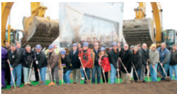
Minneapolis Building and Construction Trades leaders participate in the Vikings Stadium groundbreaking. Roofers Local 96 Business Manager Pete Jaworski is pictured far left.
