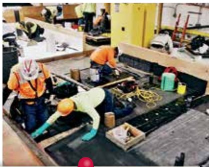
Single Ply III students work on mock-ups with EPDM and TPO as part of their final projects, installing a basic system from measurements to material list to install.
