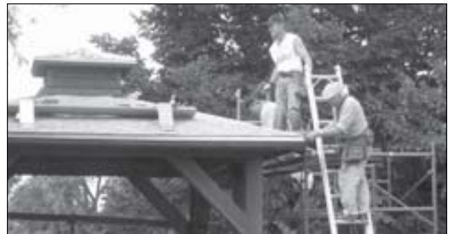
Huntz starts the ridge as Steve Schmitt, foreman at Velcheck-Finger Roof Consulting & Service, and Chris Polzin, apprentice at Standard Roofing, lay out the field.
