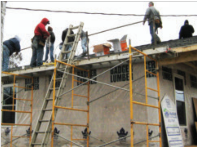
Local 242 apprentices get to work putting the roof on Wood County Habitat House #54 for the Montgomery family.
