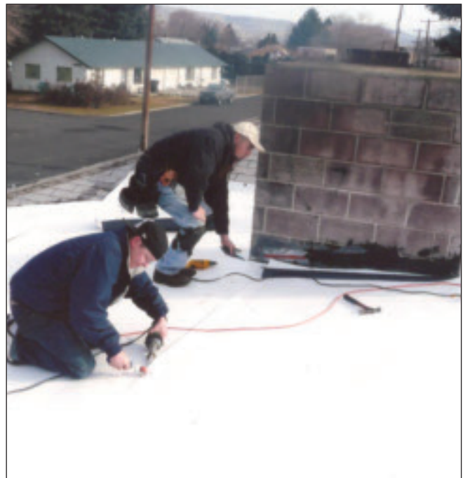
Chuck Lewis and Julio Cuevas weld seams on TPO on the Yakima job.
