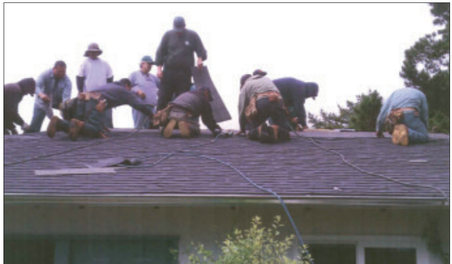
Volunteers from Local 40, San Francisco, CA, and Local 81, Oakland, CA, work together to replace a family's roof for Rebuilding Together.
