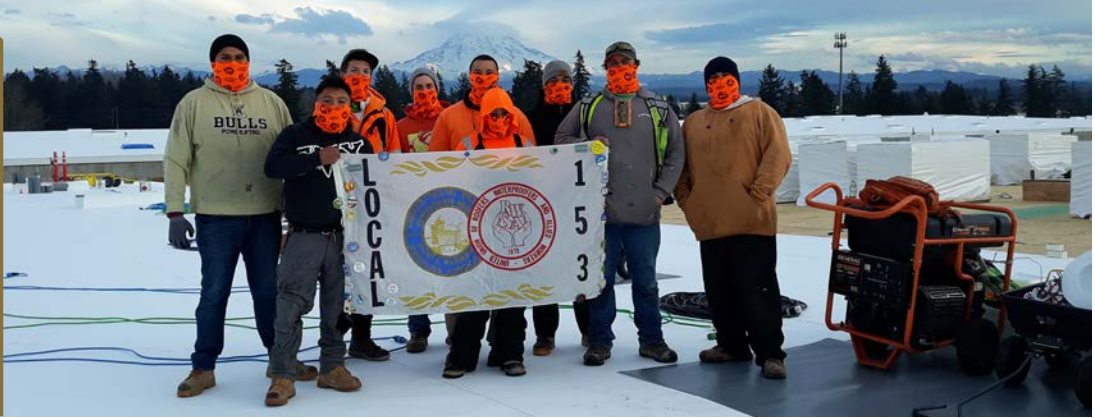
Local 153 members working for Tri-Star Roofing wrap up work on the new Big Freddy Logistics industrial development in Frederickson, WA.
